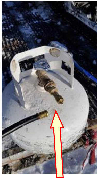
Hose broke at the tank connection when frozen
